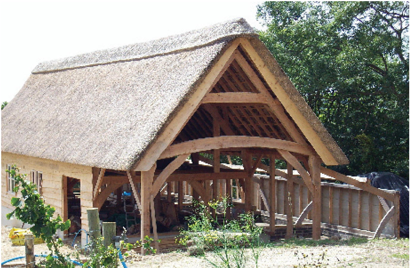
Processing room for local food at Fivepenny Farm, Wootton Fitzpaine; a timber frame building made from local Douglas fir.
